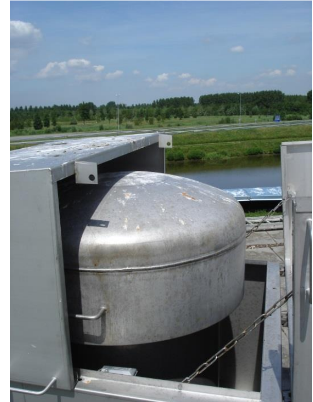
Air filter on distribution reservoir
