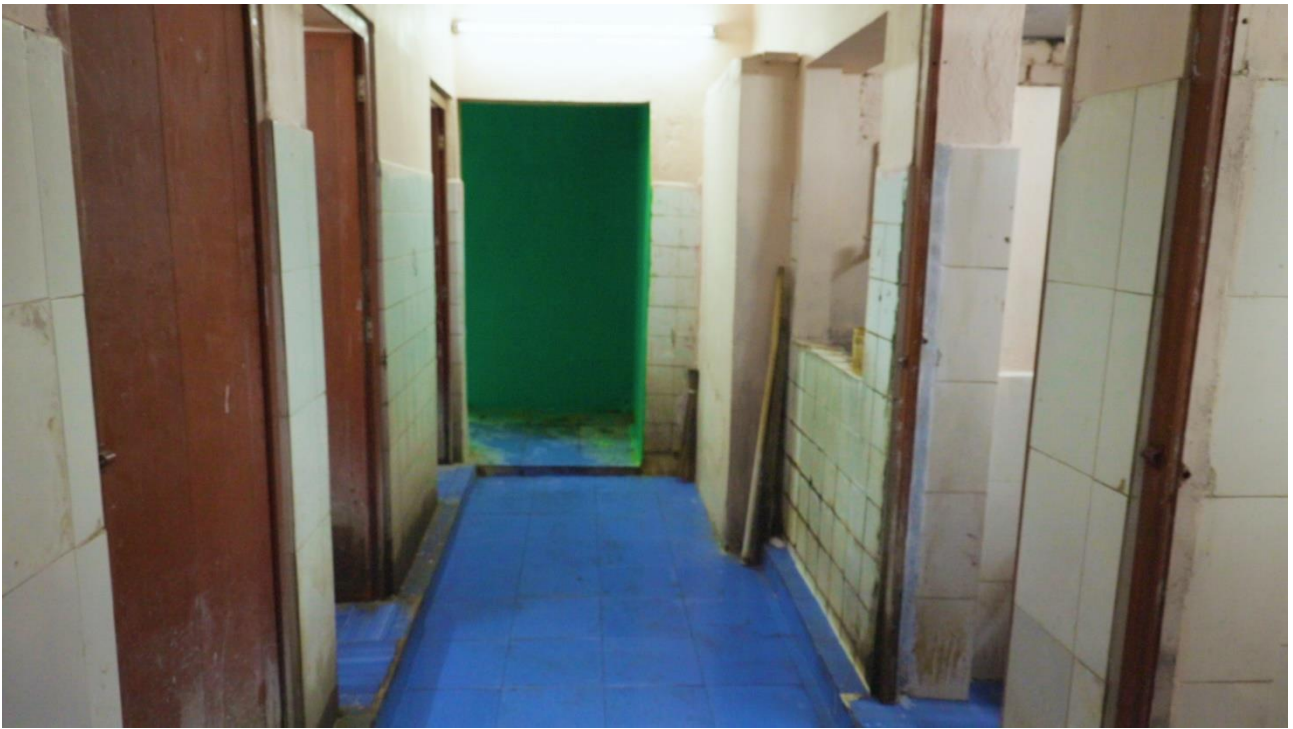
Figure 2 – Toilet facility at Thiruvanmayur, Chennai before refurbishment. Source: IIHS.
