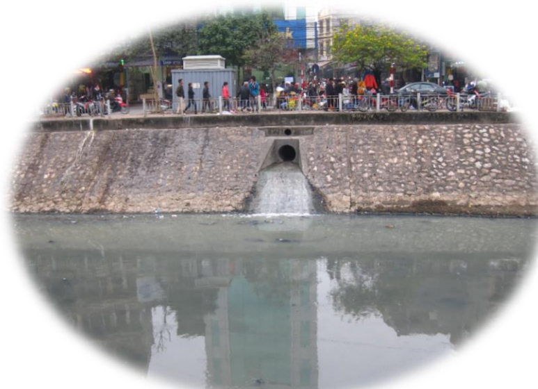
Discharge from a sewer to a river
