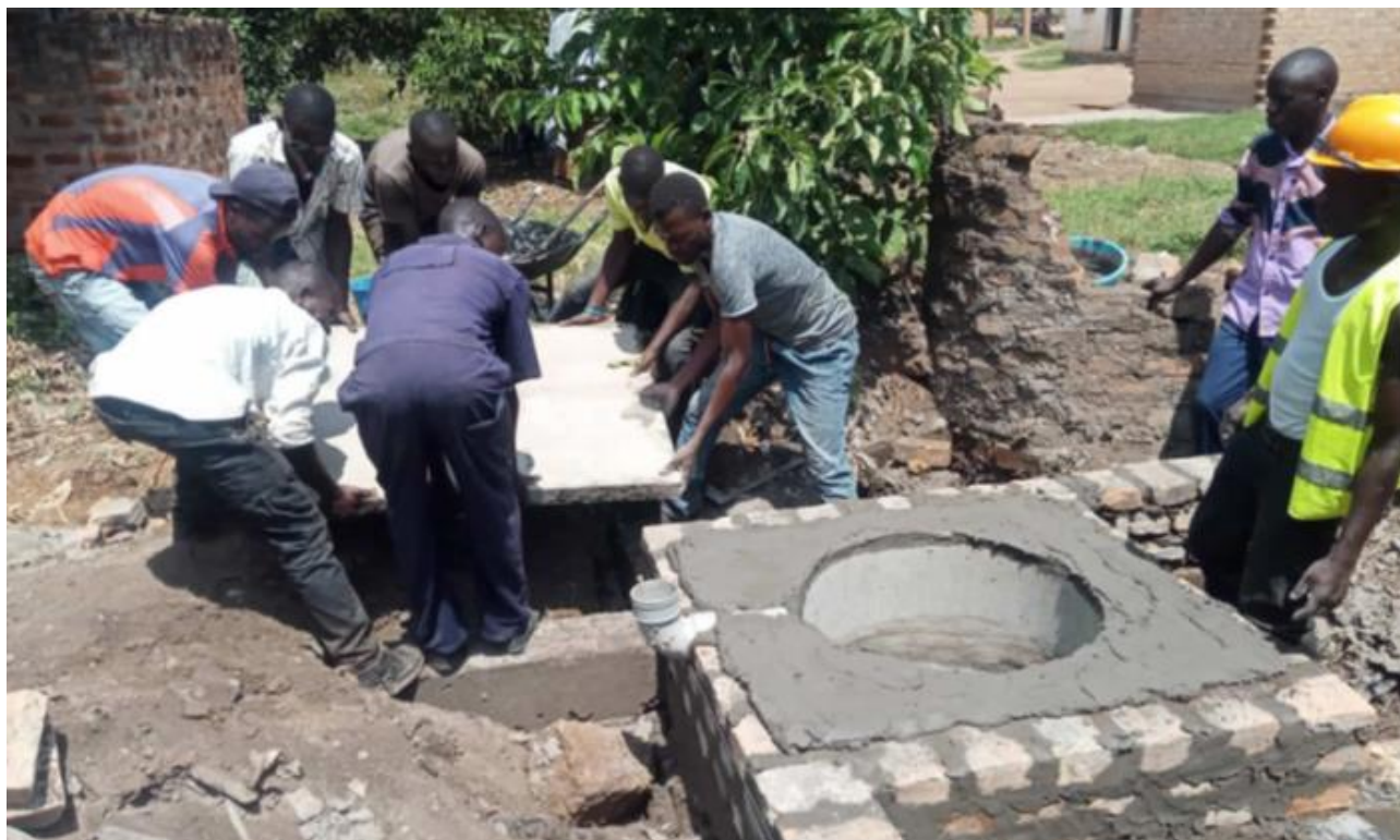
Figure 4 – Construction of toilet substructures at a household in Apac. Source: GIZ – Sanitation for Millions.
