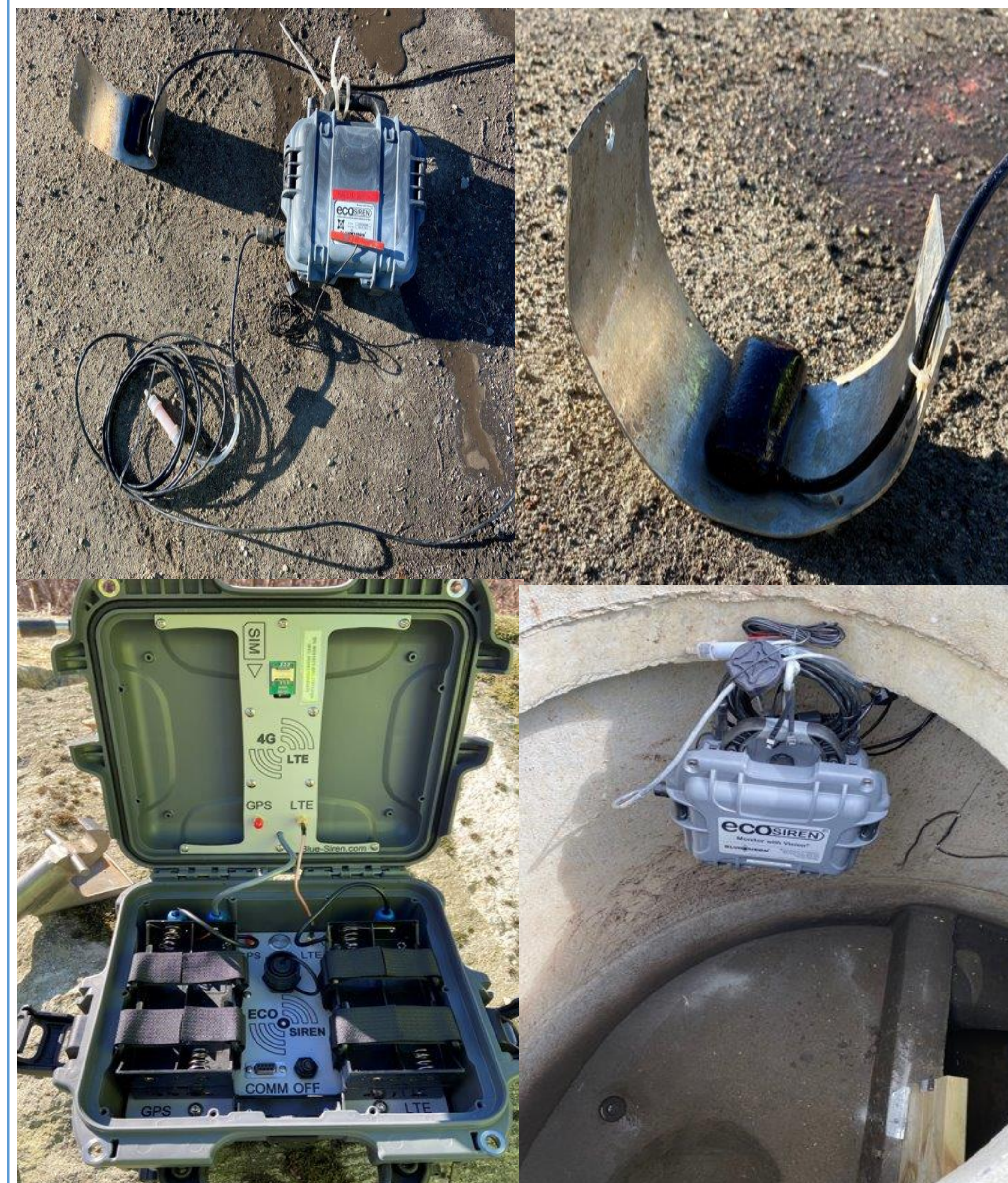
Figure 1: Water amount sensor connected to a 4G internet network and installed in a manhole.
